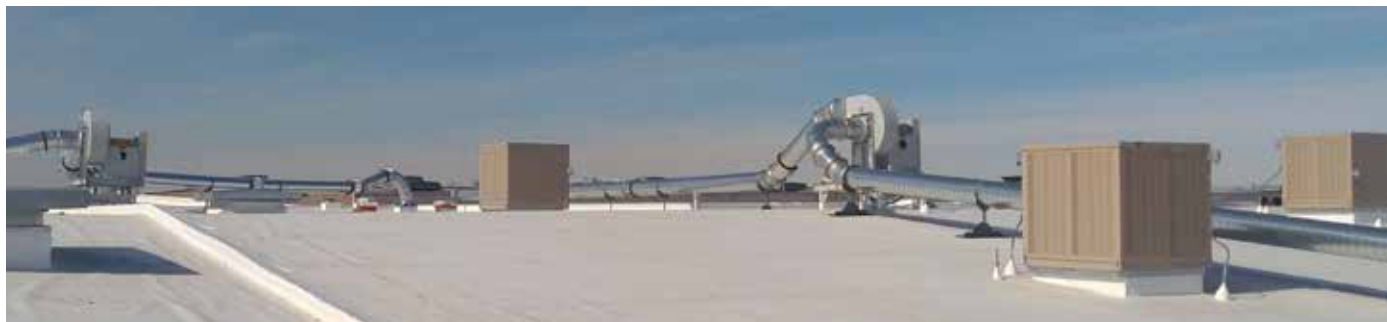
The above roof duct and blower system at Wasatch Container was installed by G.F. Puhl
